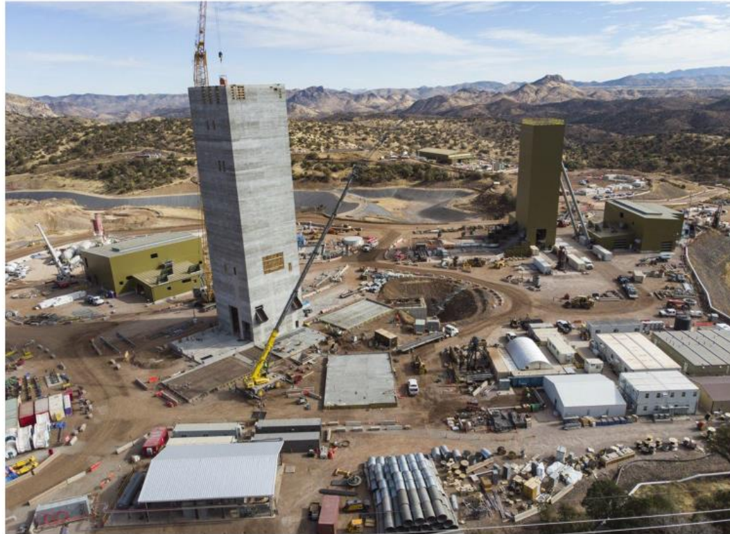
Construction of main shaft (left), ventilation shaft (right) and tailings storage (rear)
